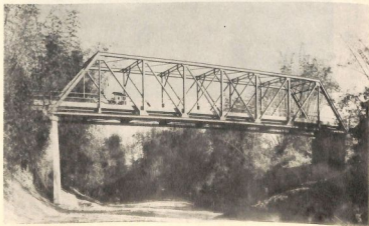
61. Single steel truss bridge, 195' x 16' x 30', on Route 5B over Tabuating R. near Sta. Rosa, Nueva Ecija. Pre-war.
