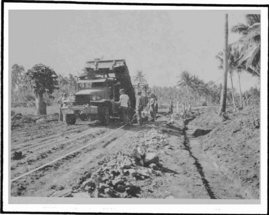
Drainage became the major engineering problem during the January 1945 heavy rains. The existing highway No.1, (north of ABUYOG)
